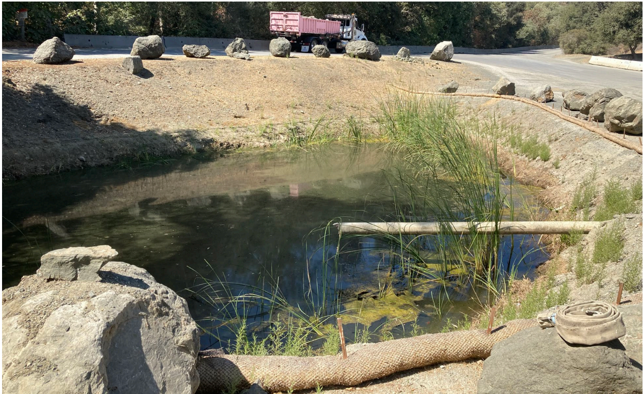
Photo 30: Settling basin near main entrance.
