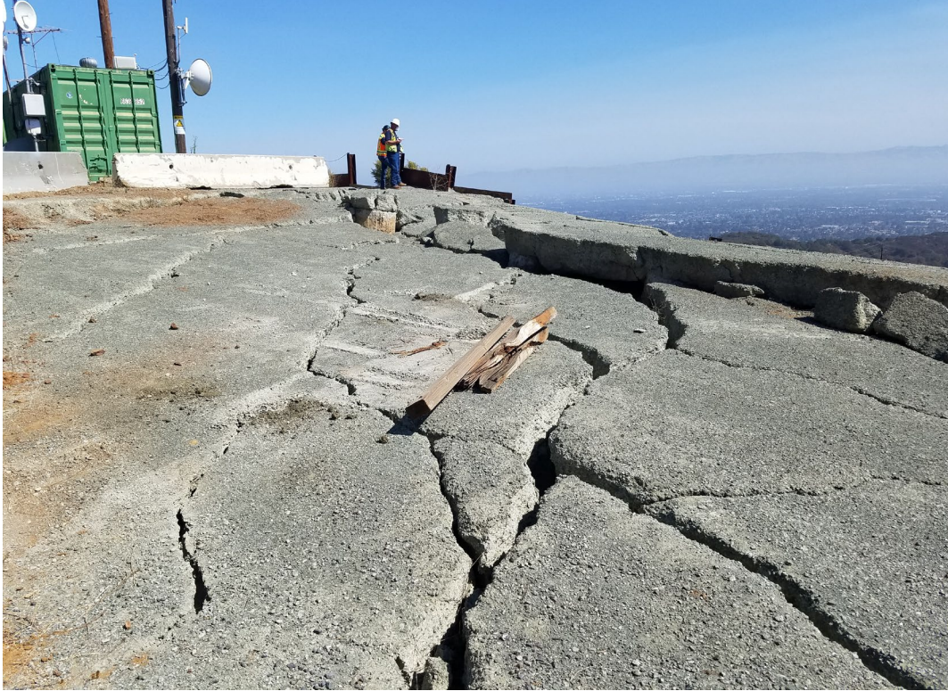
Photo 17: Ground cracks near northwest property line.
