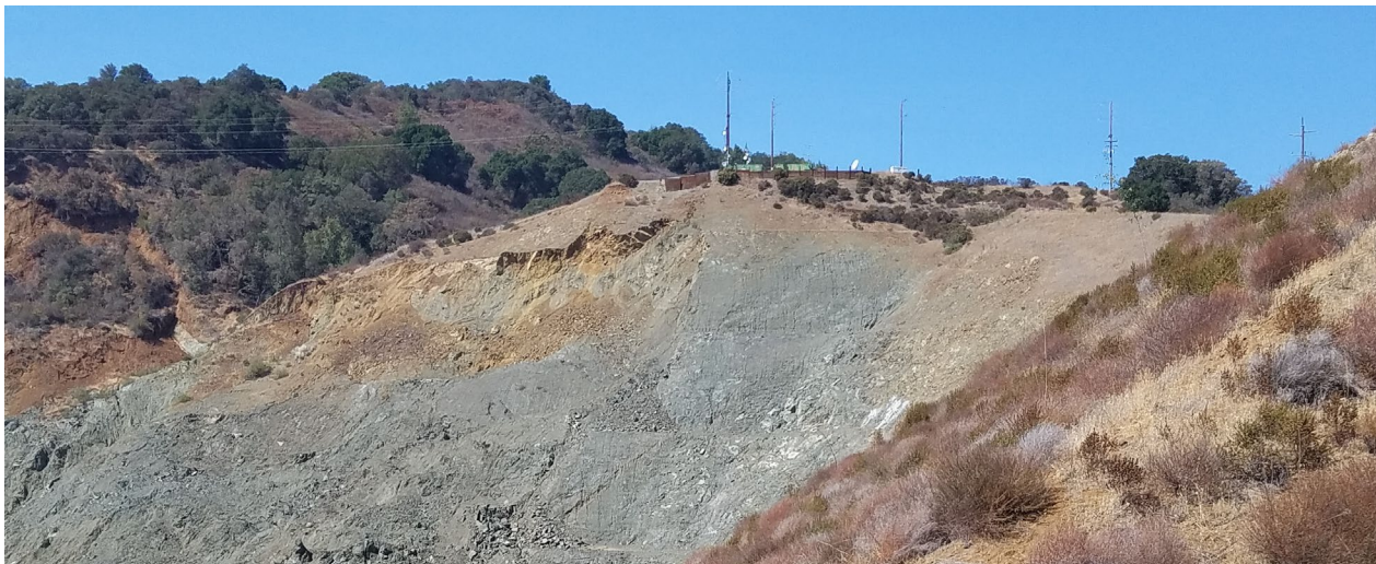
Photo 1516: Slope failure on western high cut wall.
