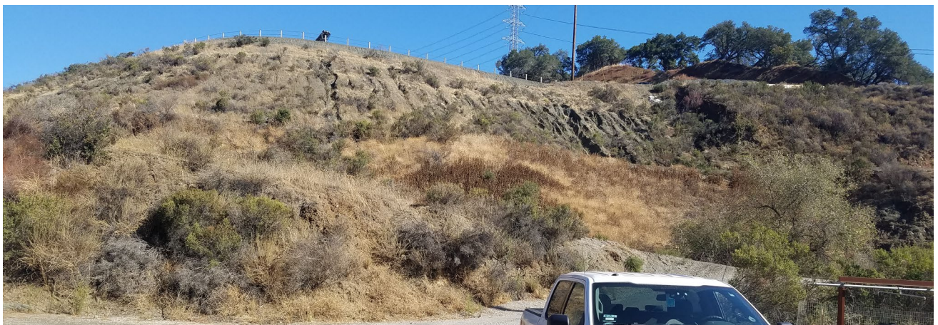
Photo 7: Erosion rills on fill slope above main haul road.
