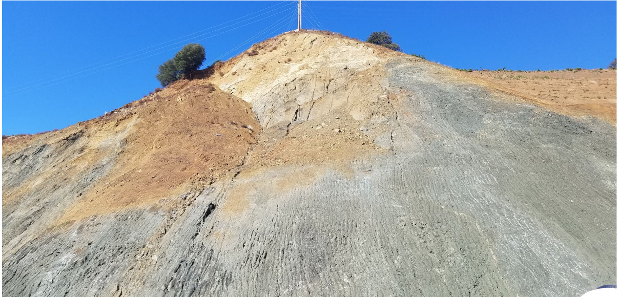
Photo 20: Slope failure on southwestern high cut wall below three PG&E poles, looking west.
