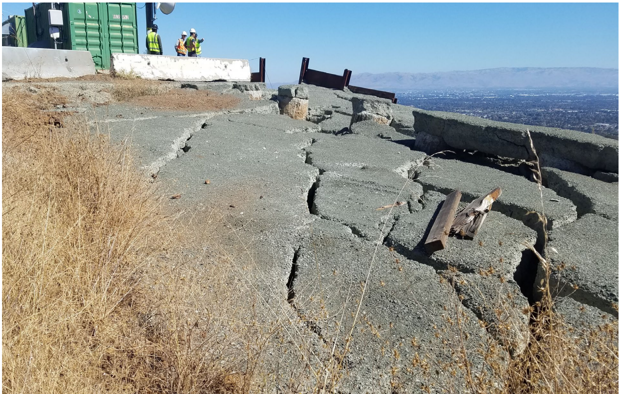
Photo 17: Ground cracks near radio containers at northwest property line.
