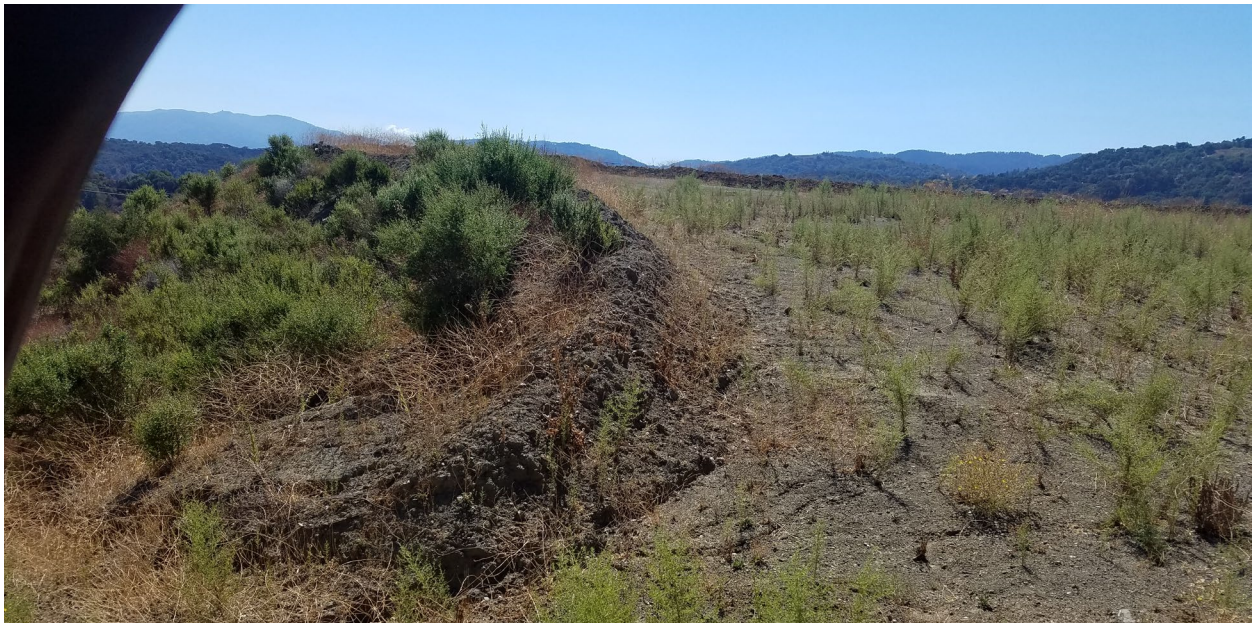
Photo 11: Regraded area where ground cracks on top of buttress fill of north high wall were observed during 2020 inspection.
