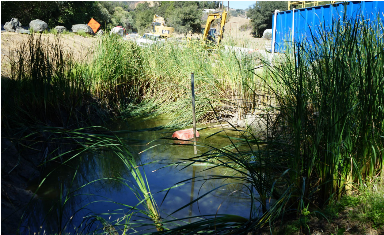
Photo 30: Settling basin near main entrance.
