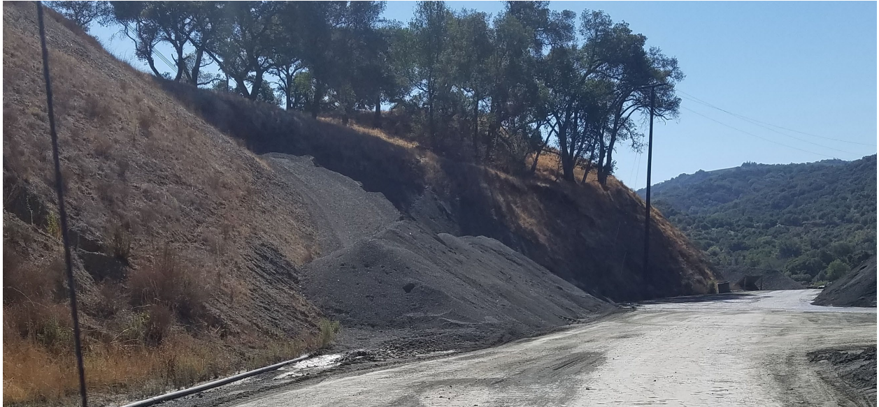
Photo 22: Shallow failures of cut slope along east side of Parcel B (in tree shadows).
