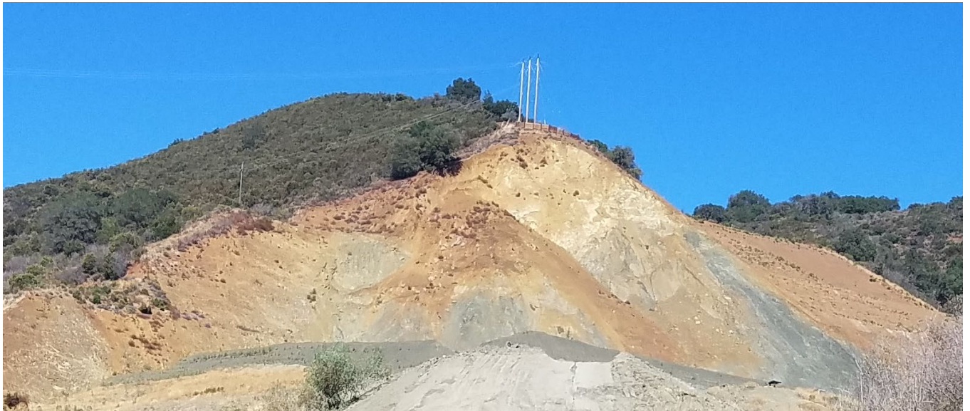
Photo 19: Slope failure on southwestern high cut wall, looking south. (Profile view)
