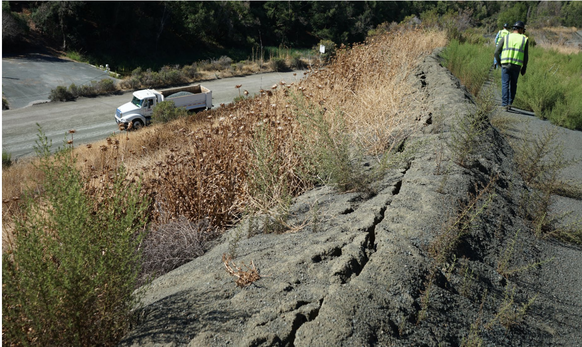
Photo 35: Open crack in fill berm and non-native weeds located along south side of graded road above main haul road.
