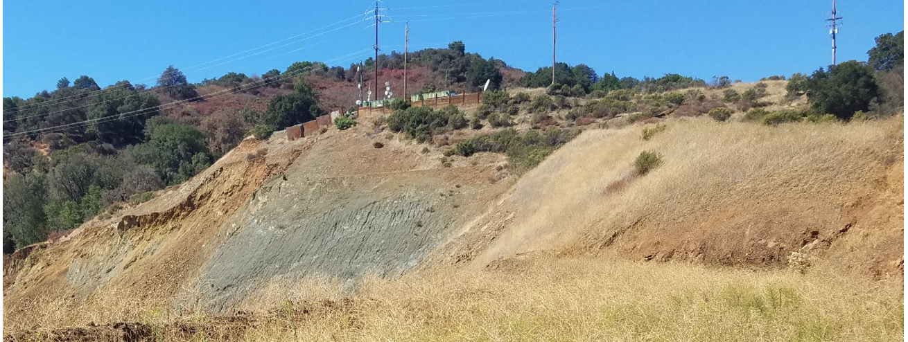
Photo 1516: Slope failure below radio containers on western high cut wall.
