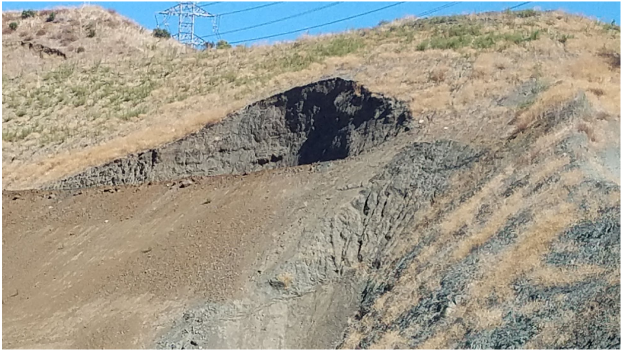
Photo 33: Slope failure scar (debris removed) located near the northeastern corner of Parcel B.
