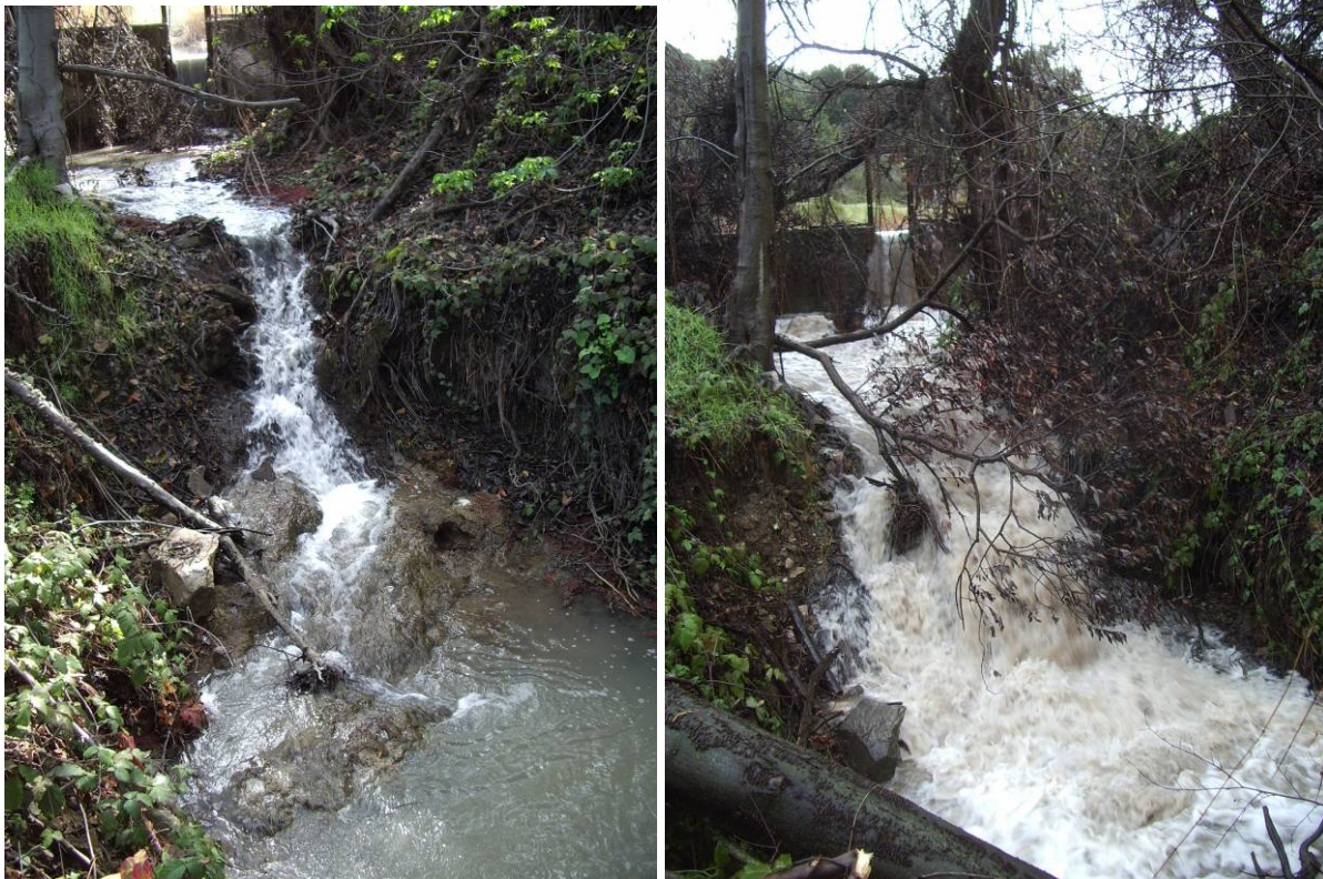
Figure 2-12 Headcut downstream of the Pond 14 weir
