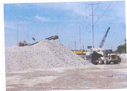
Recycled crushed concrete being loaded into a semi-dump truck to be used as granular fill.
