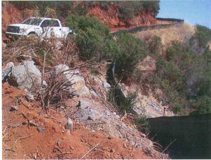
Photo 13: Silt fence BMP along outer edge of mid-slope bench in southern slope of WMSA required by regrading the roadway for the installation of groundwater monitoring wells. Dated September 3, 2015.
