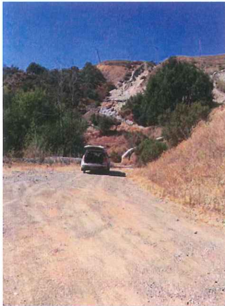
Photo 25: Looking northwest from the area of Pond 13B at the washed out slope caused by overflow of the new crusher sump in December 2014. Dated September 3, 2015.
