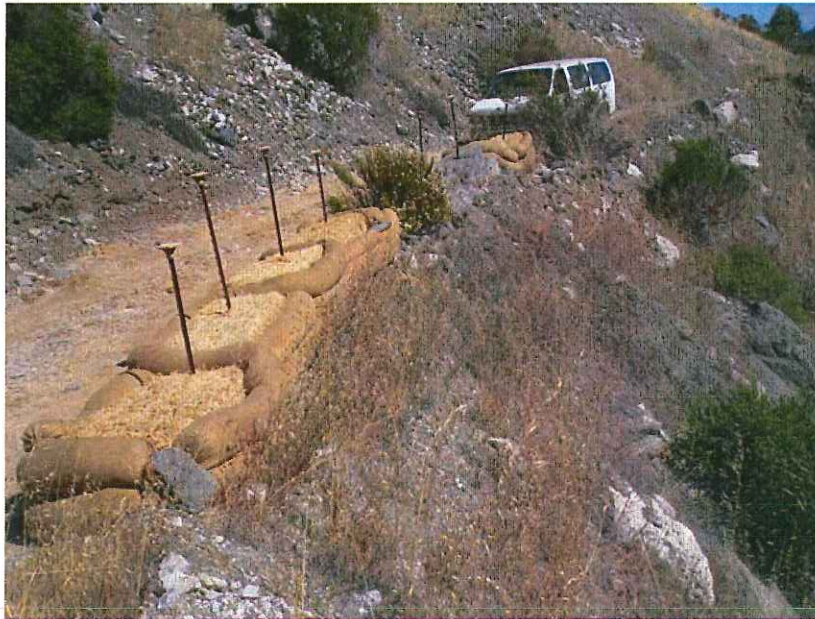
Photo 7: Straw waddle and haybale BMPs placed along mid-slope bench roadway in southern WMSA slope. Dated September 3, 2015.
