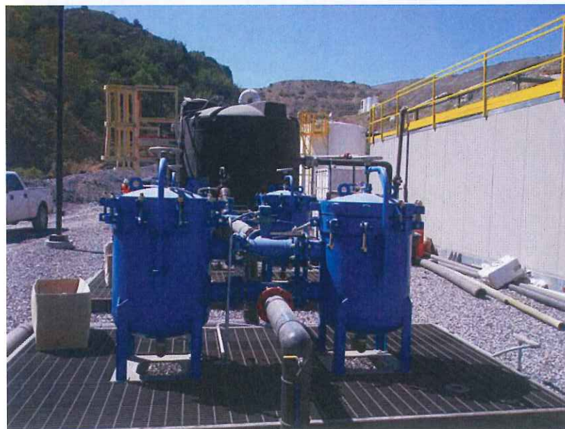
Photo 34: Interim treatment plant south of the North Quarry, looking west. Dated September 3, 2015.
