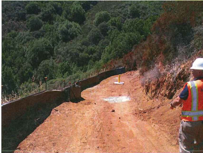
Photo 11: Silt fencing on mid-slope bench roadway at western end showing protective riser for groundwater monitoring well. Dated September 3, 2015.
