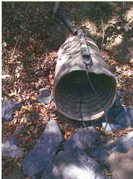
Photo 20: Pond 30 metered outfall to Permanente Creek. Dated September 3, 2015
