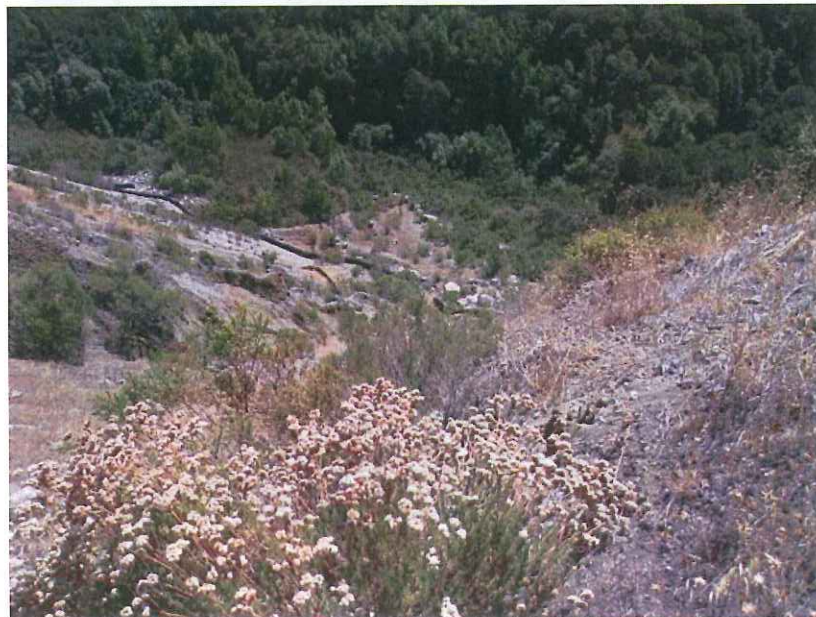
Photo 10: Silt fencing on southern slope of WMSA below mid-slope bench; silt fencing shows no visible significant displacement. Dated September 3, 2015.
