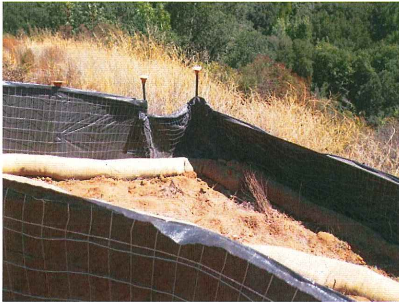
Photo 12: Silt fence and straw waddle BMPs along outer edge of mid-slope bench in southern slope of WMSA required by regrading the roadway for the installation of groundwater monitoring wells. Dated September 3, 2015.
