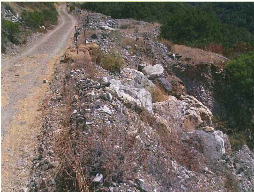
Photo 8: Rocked outfall in mid-slope bench on southern WMSA slope, looking southwest. Dated September 3, 2015.
