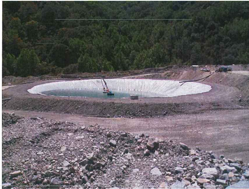
Photo 35: Looking south at the new lined pond south of the North Quarry that holds water for discharge to the interim treatment plant shown in Photos 33 and 34. Dated September 3, 2015.
