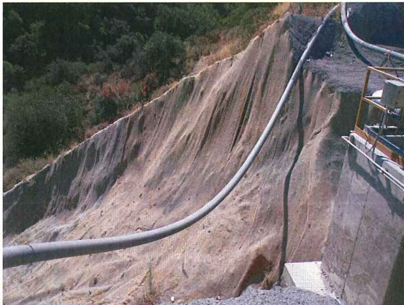
Photo 24: Upper portion of slope washed out by overflow of crusher sump. Sump wall exposed in lower right of image, looking west. Slope repair will need to underpin foundation of sump. Dated September 3, 2015.
