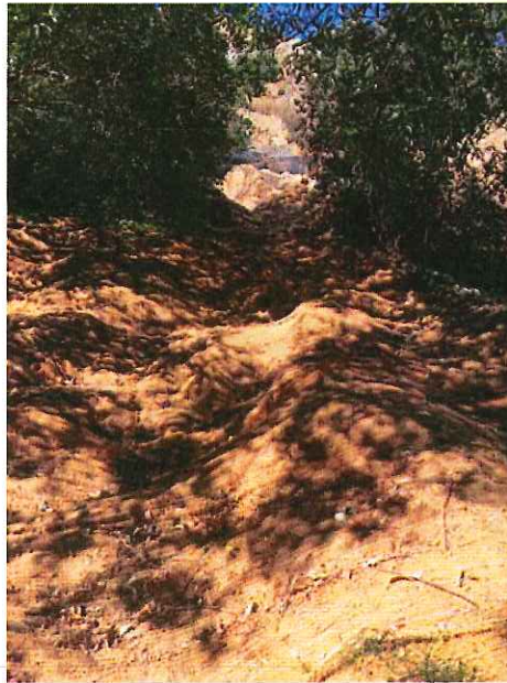
Photo 27: Lower portion of washed out slope caused by overflow of the new crusher sump in December 2014. Material discharged into Pond 13B. Dated September 3, 2015.
