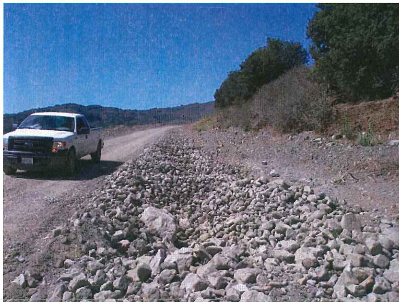
Photo 15: Non-limestone drainage channel/French drain on inside of main roadway in EMSA looking south. Drain discharges into channel shown in Photo 16. Dated September 3, 2015.
