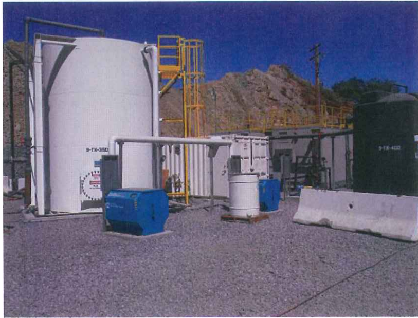
Photo 33: Interim treatment plant at south of North Quarry. Plant discharges to Pond 4A and then to Permanente Creek. Plant wasn't operating at time of 2015 inspection because all water was being used in mining operations. Dated September 3, 2015.
