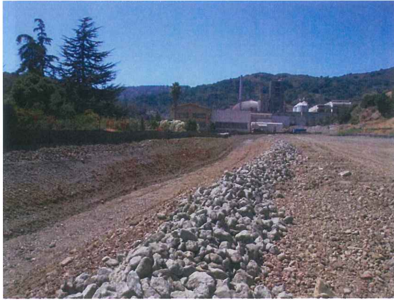
Photo 17: Looking south at drainage channel that flows northward to discharges EMSA stormwater into Pond 30. Dated September 3, 2015.
