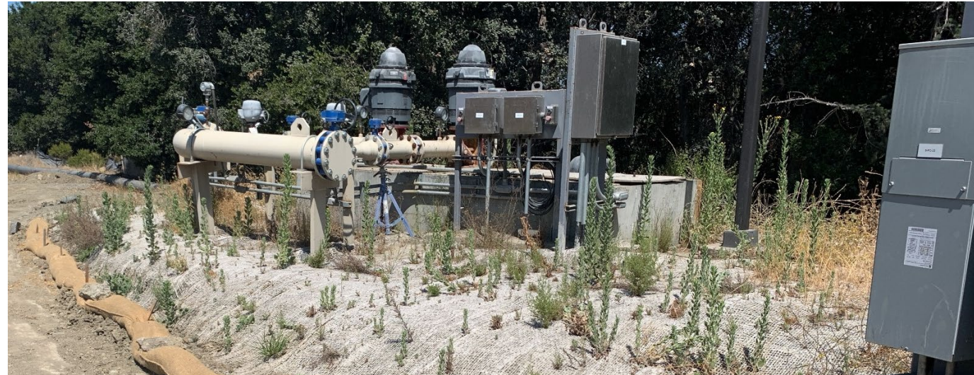
PHOTO #9A – Vault and pump at Pond 30
