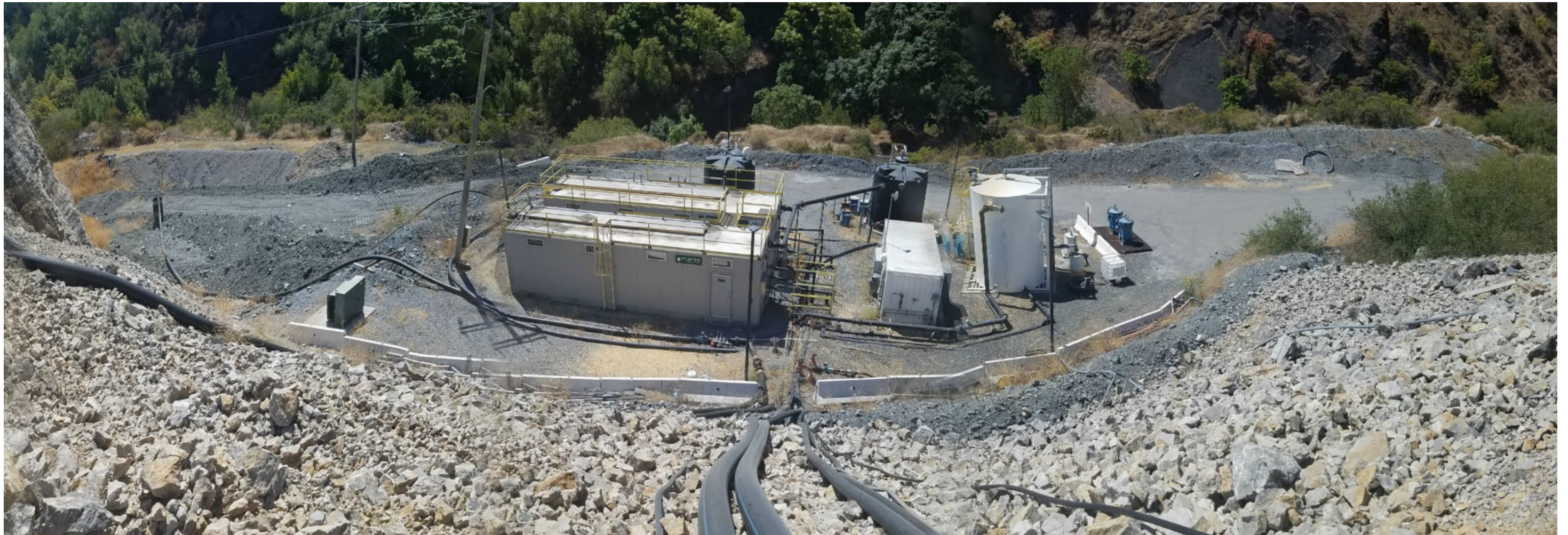
Adjacent to Pond 4A are water treatment and filtration equipment used to remove selenium from quarry water prior to discharge into Permanente Creek. [See PHOTO #18.]
