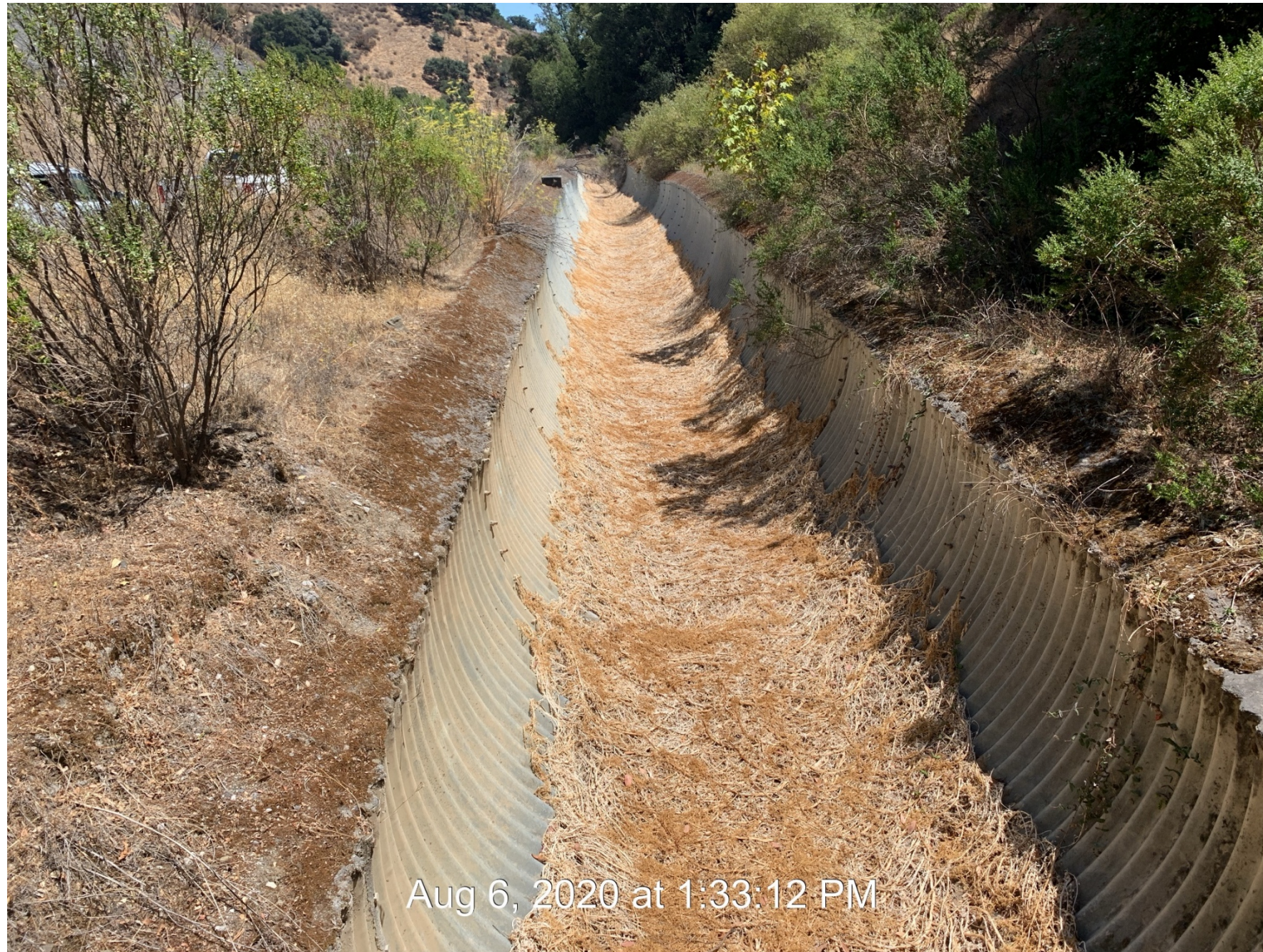
A half-pipe exists downstream of Pond 13 for the continuance of Permanente Creek. [See PHOTO #12. ]
