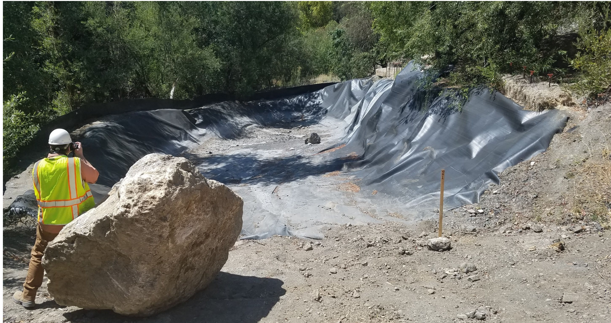
Photo #26 – Debris basin
