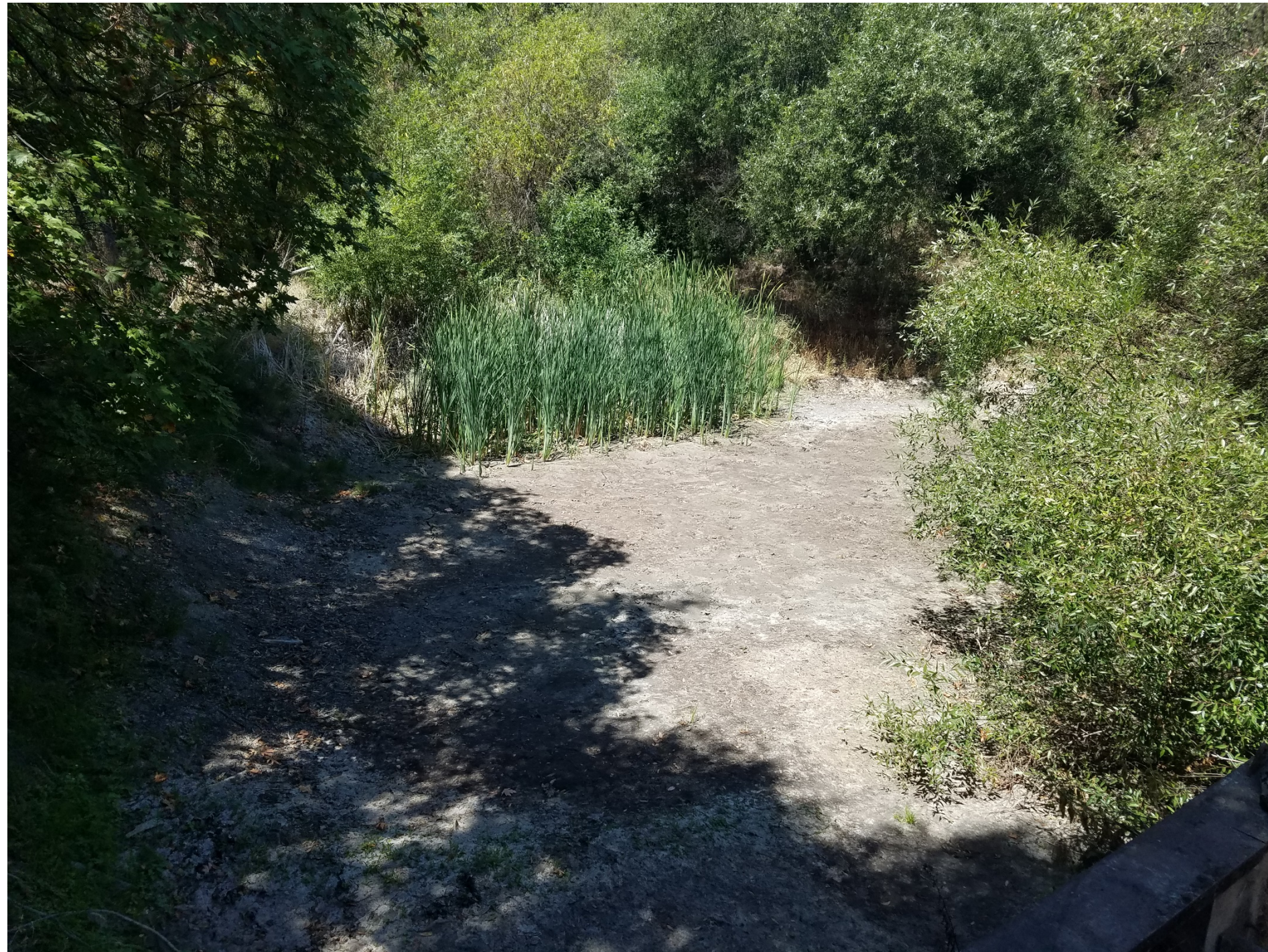
Eroded material accumulated at the toe of the slope and extended into the eastern side of Pond 13. [See PHOTO #11 ]
