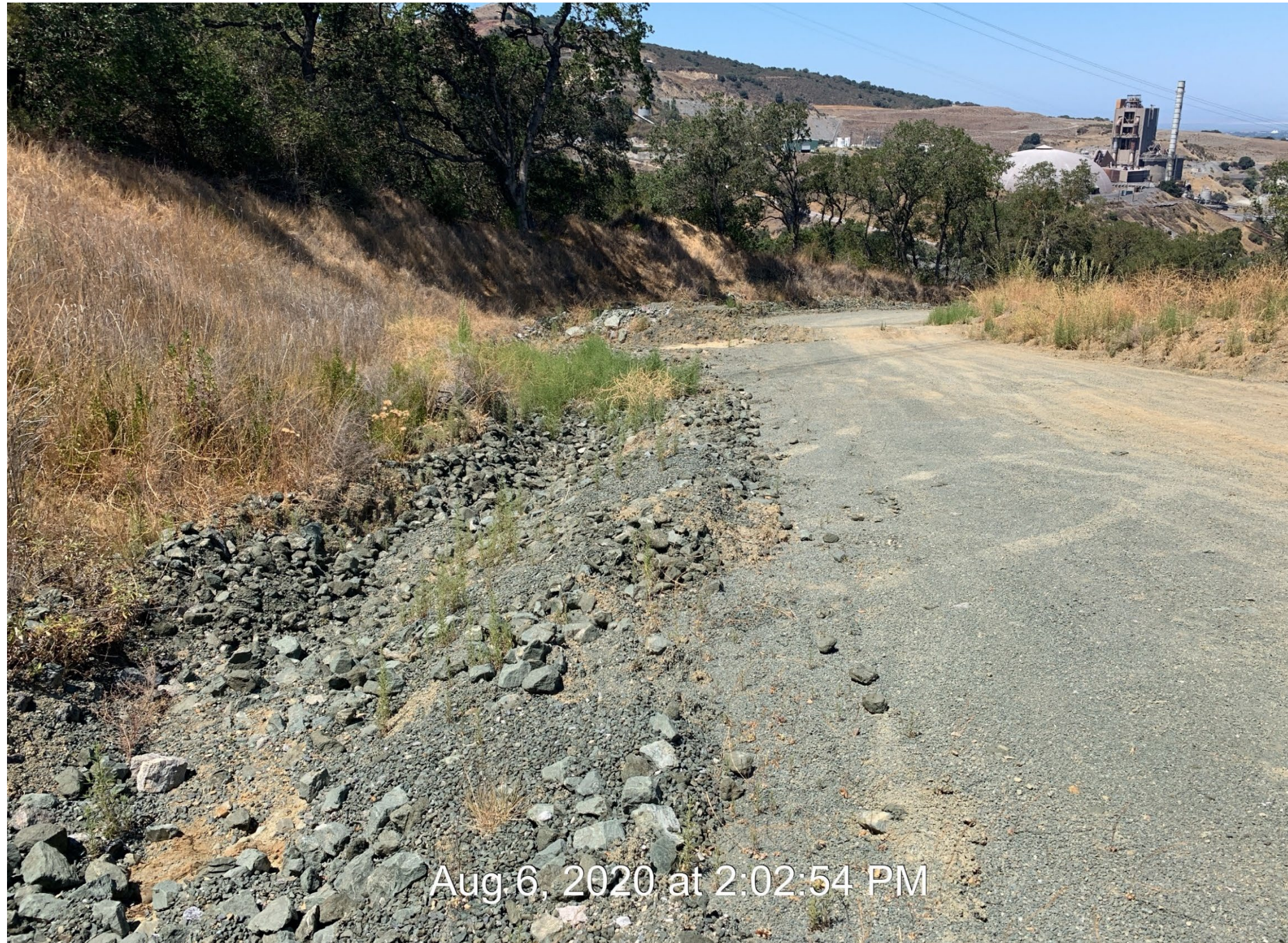
Photo #21A – Cut slope and drainage ditch on west side of illegally graded haul road
