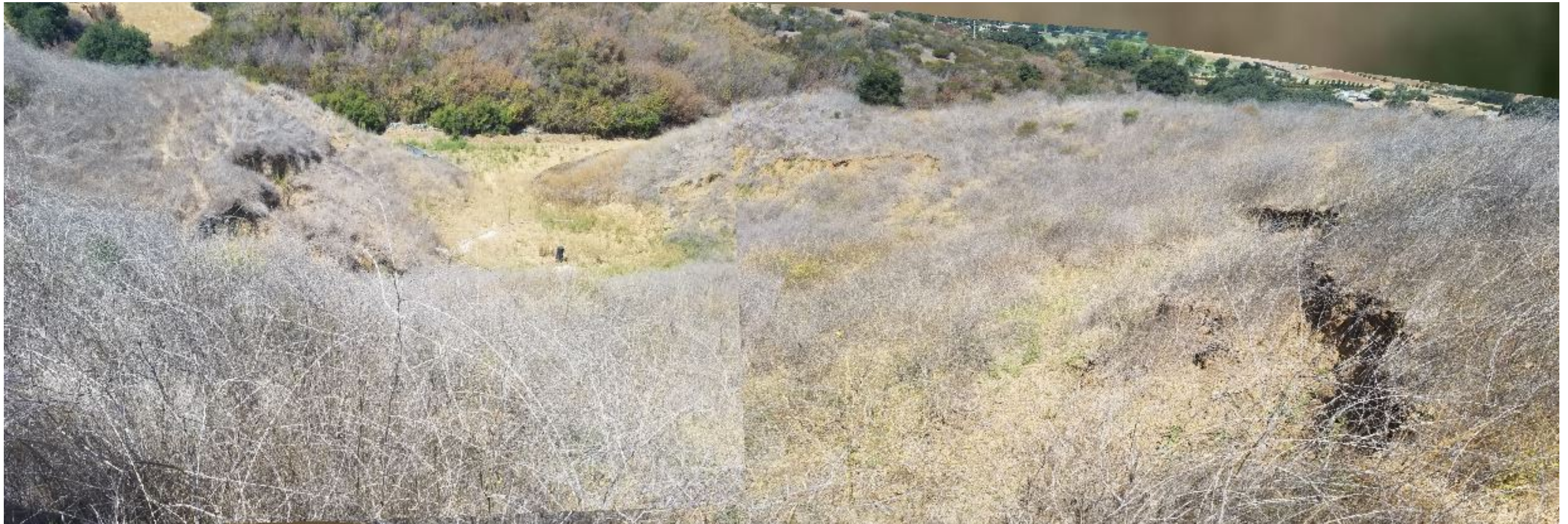
Photo #29 – Shallow slumps in fill material added to EMSA beginning in September or October of 2017
