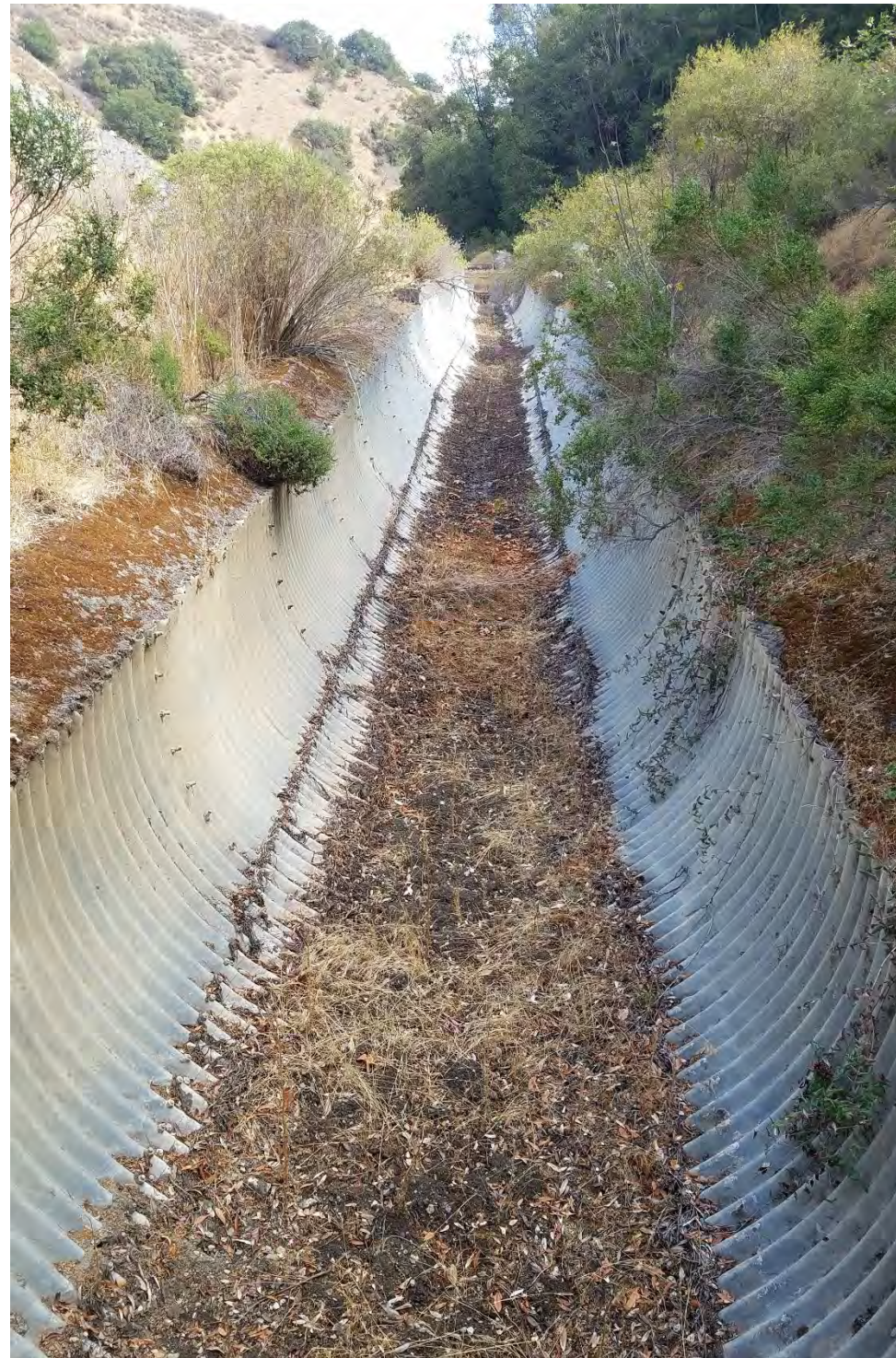
PHOTO #12 – Half-pipe for outflow of Pond 13
