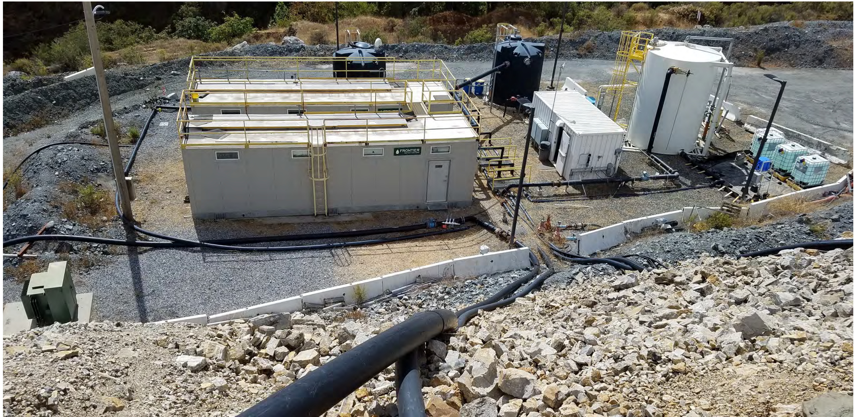
Adjacent to former Pond 4A is water treatment and filtration equipment used to remove selenium from quarry water prior to discharge into Permanente Creek.
