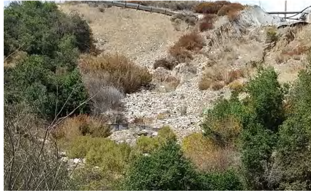
PHOTO #10A – Overflow scar below crusher sump
