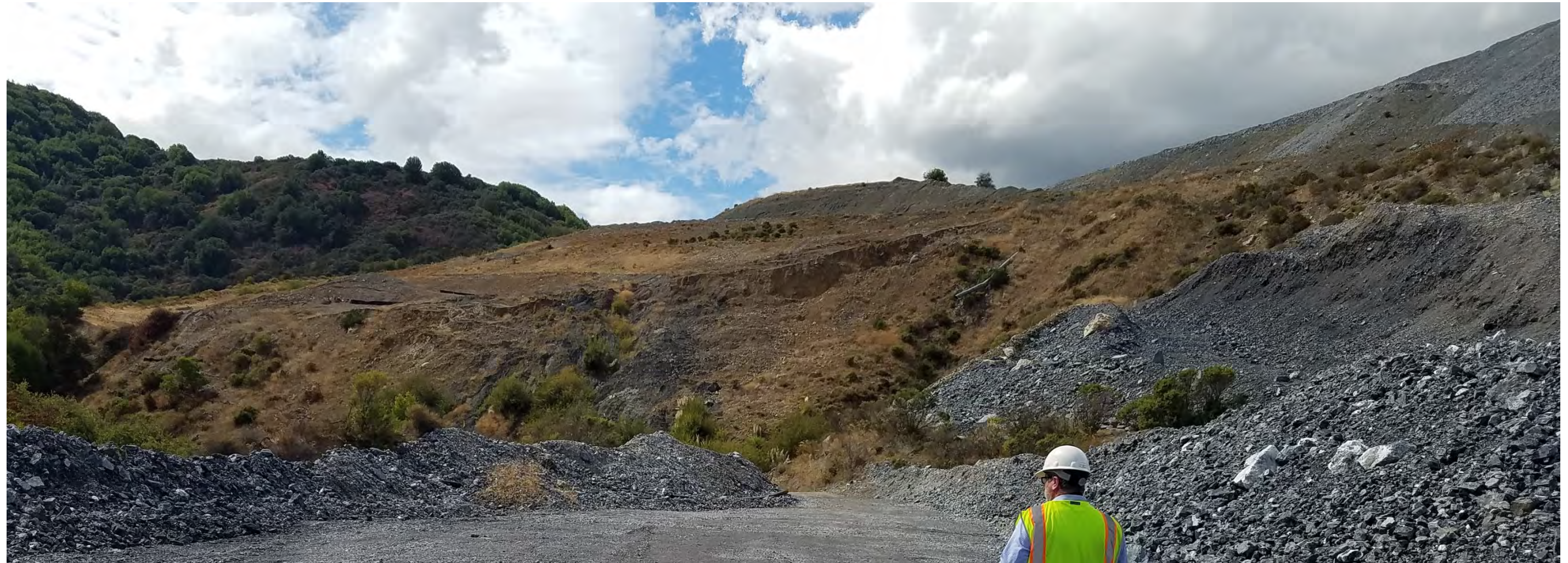
Photo #24 – Toe of Yeager Yard landslide above Permanente Creek (lower left)
