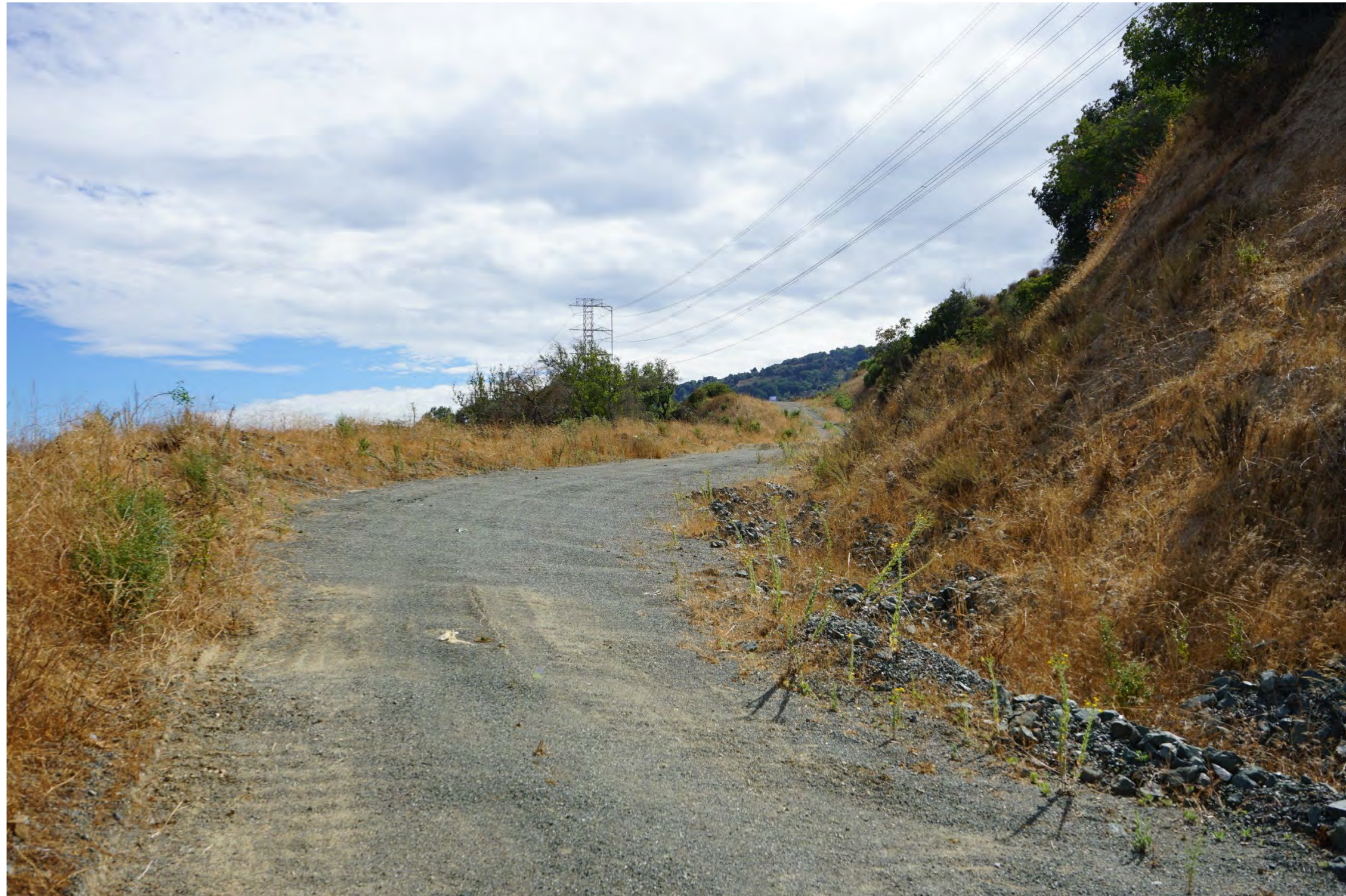
Photo #21A – Cut slope and drainage ditch on west side of unpermitted haul road
