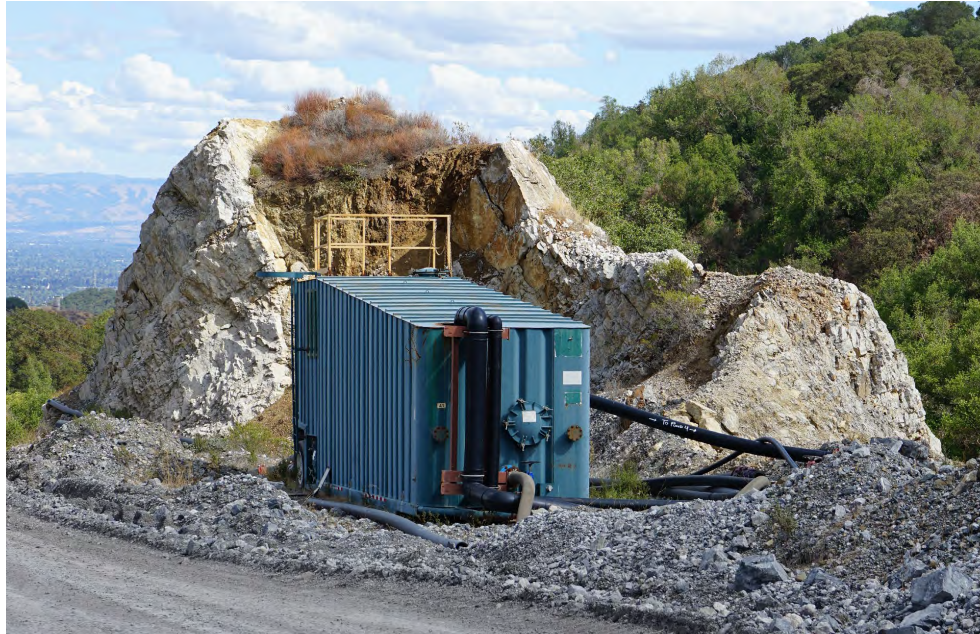
Map Location 7: Water Treatment Facilities
