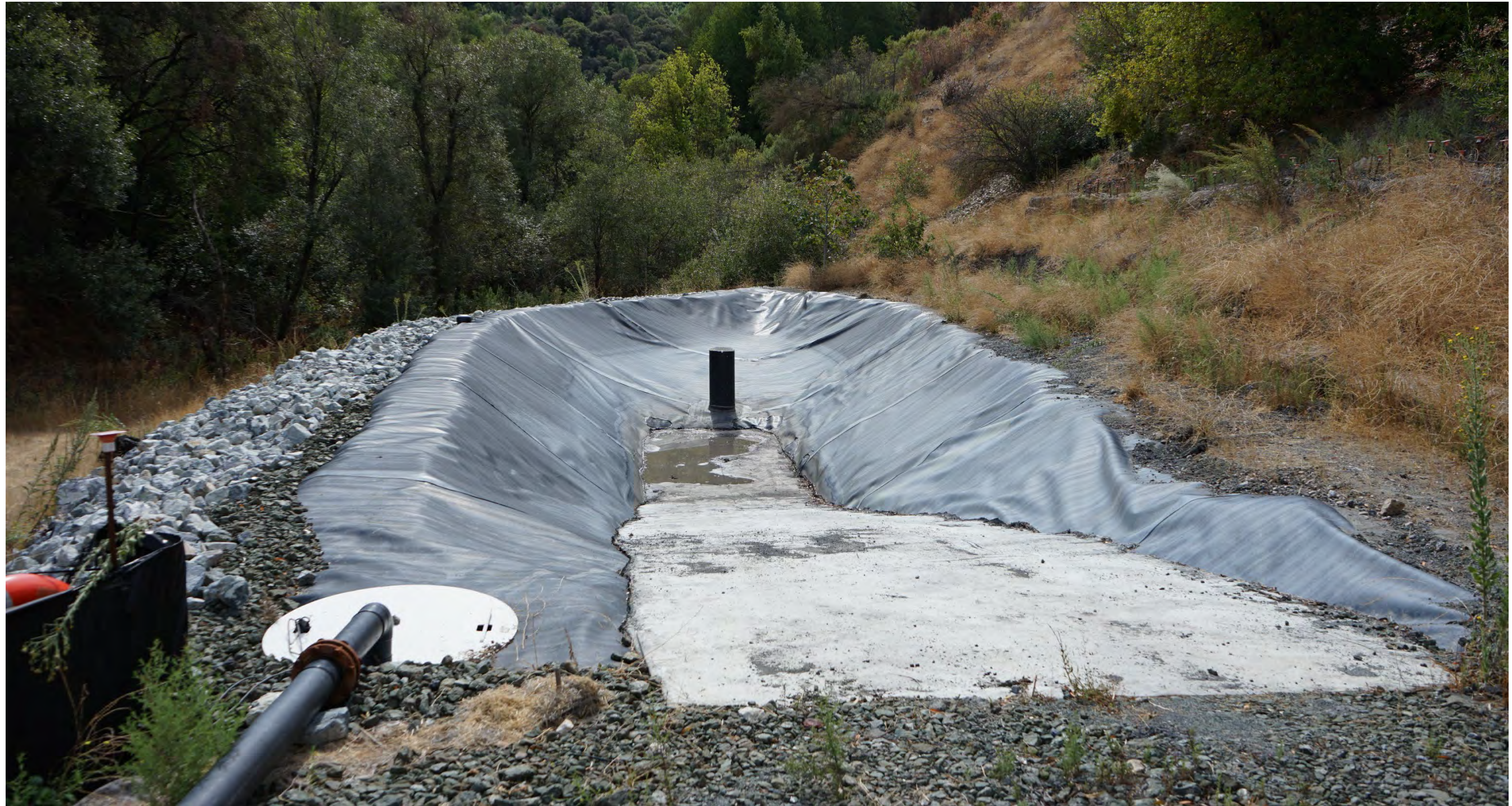
Photo #26 – Debris basin
