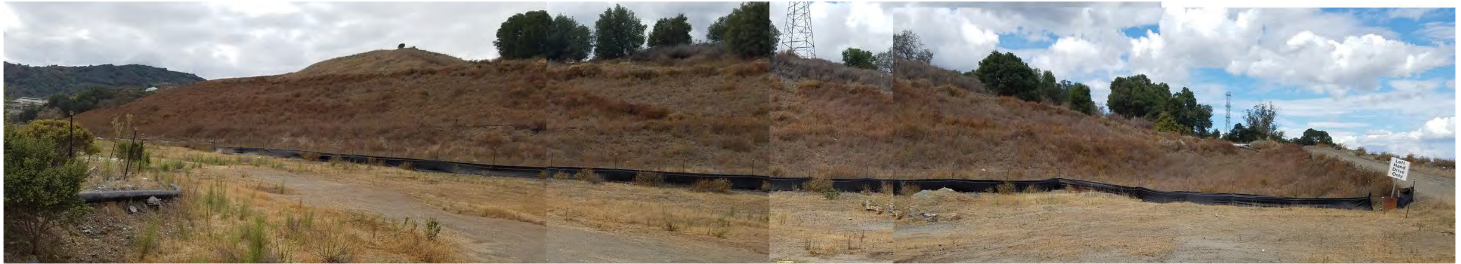
County inspectors observed substantial vegetation growth on the EMSA slopes.
