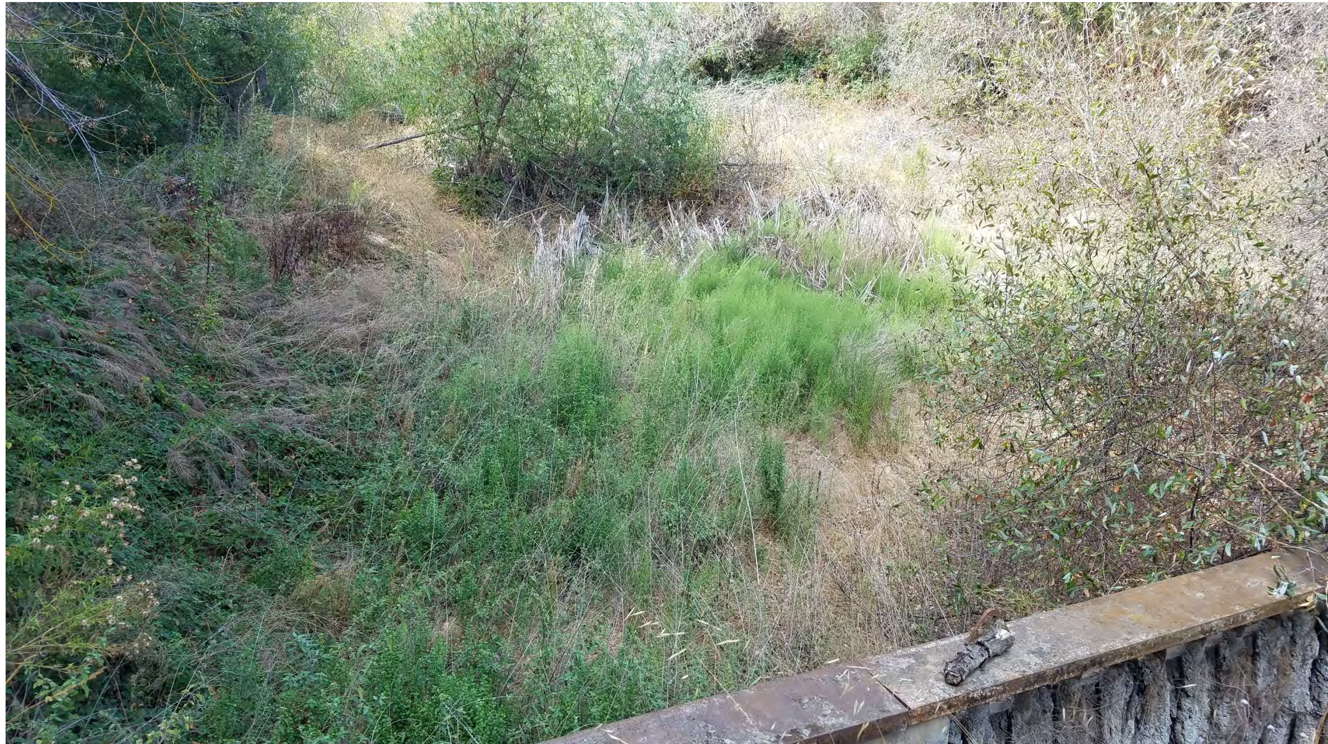
Eroded material accumulated at the toe of the slope and extended into the eastern side of Pond 13.
