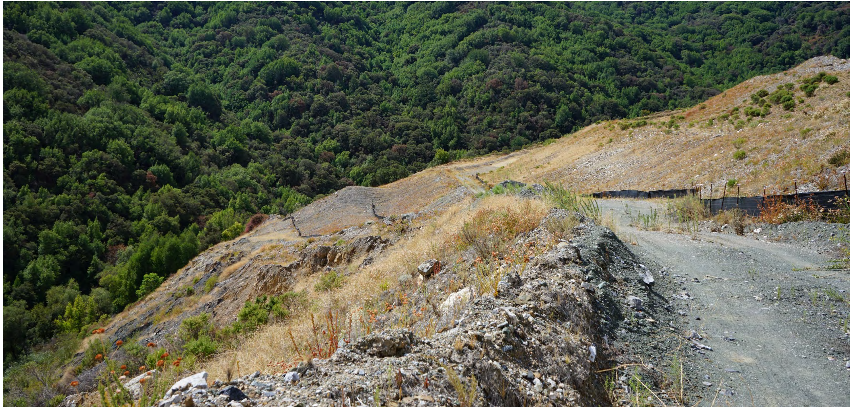
Photo #22 – Toe of Yeager Yard slide above Permanente Creek (out of view to the left)
