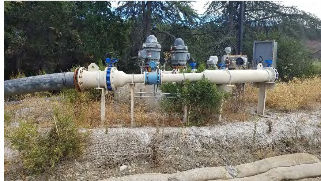
PHOTO #9A – Vault and pump at Pond 30
