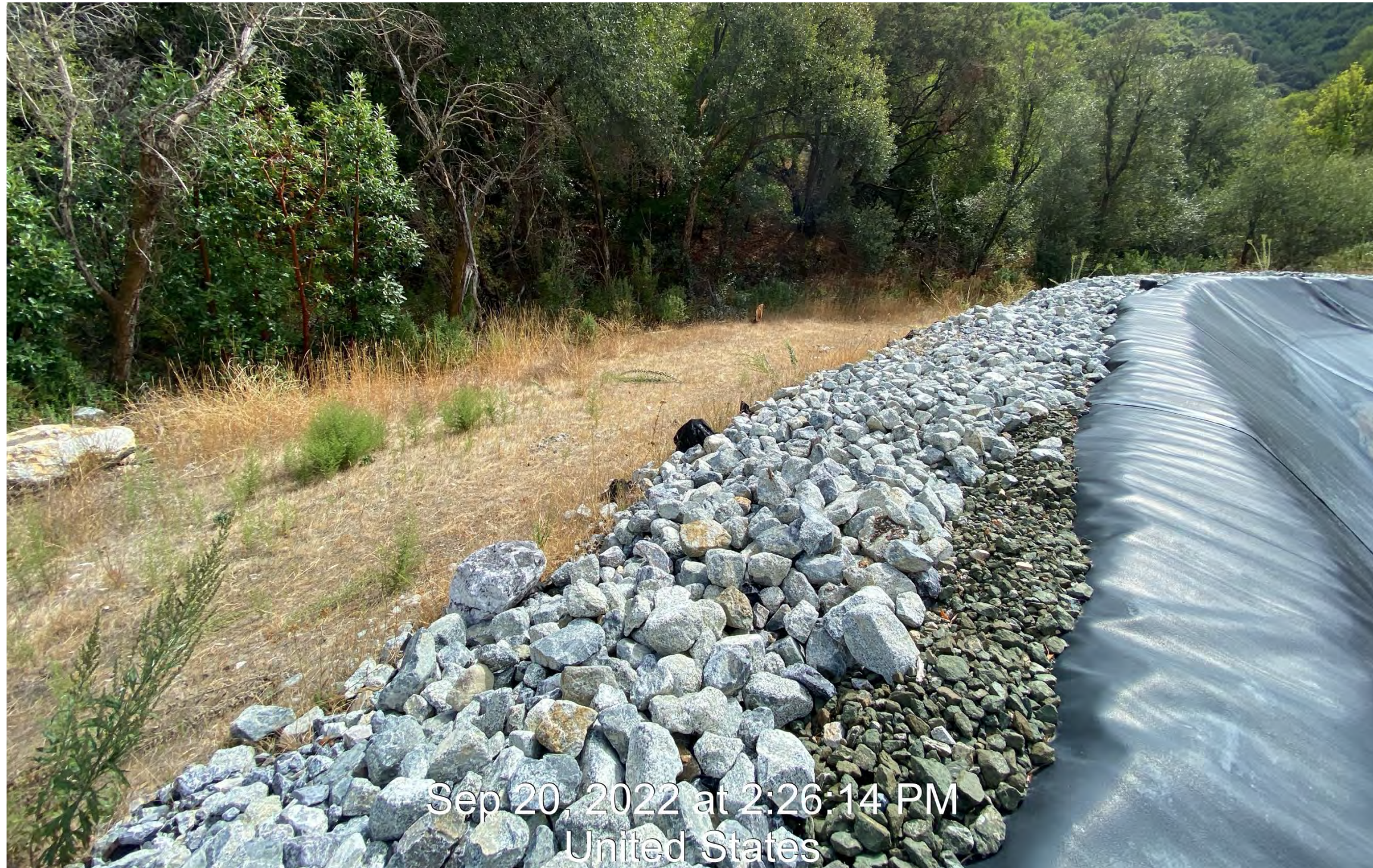
Photo #25 – Rock armor added to area where sediment was deposited into Permanente Creek from Yeager Yard slope
