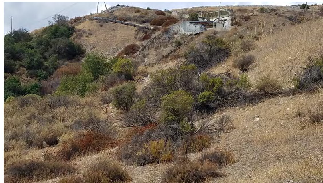
PHOTO #10B – Debris flow track below crusher
