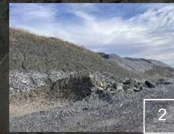
2 Water bars were established, and check dams were cleared of sediment along the WMSA Haul Road.
