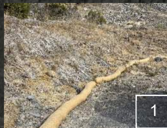
1 Straw wattles were installed at the vicinity of the sediment basin at Yeager Yard.
