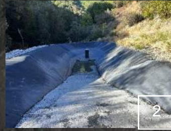
Sediment capture basin is largely clear of sediment at the base of the Yeager Yard.
