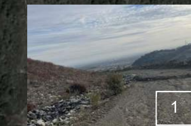
1 Water bars along EMSA Access Road were reestablished and are in functional condition.
