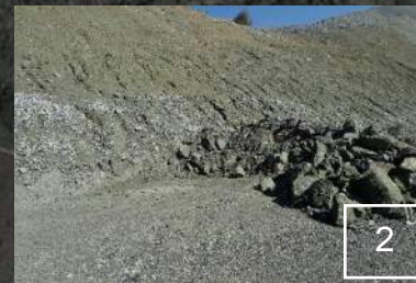
Water bars were reestablished, and check dams were cleared of sediment along the WMSA Haul Road.
