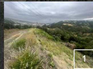
Vegetative cover is invigorated where sloughing was observed throughout the quarry during this rain season.
