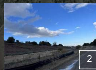
2 Silt fence fabric along the EMSA access road was repaired and is in functional condition.
