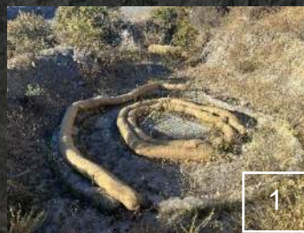
Hay bales and straw wattles were replaced at drop inlet by the EMSA access road.
