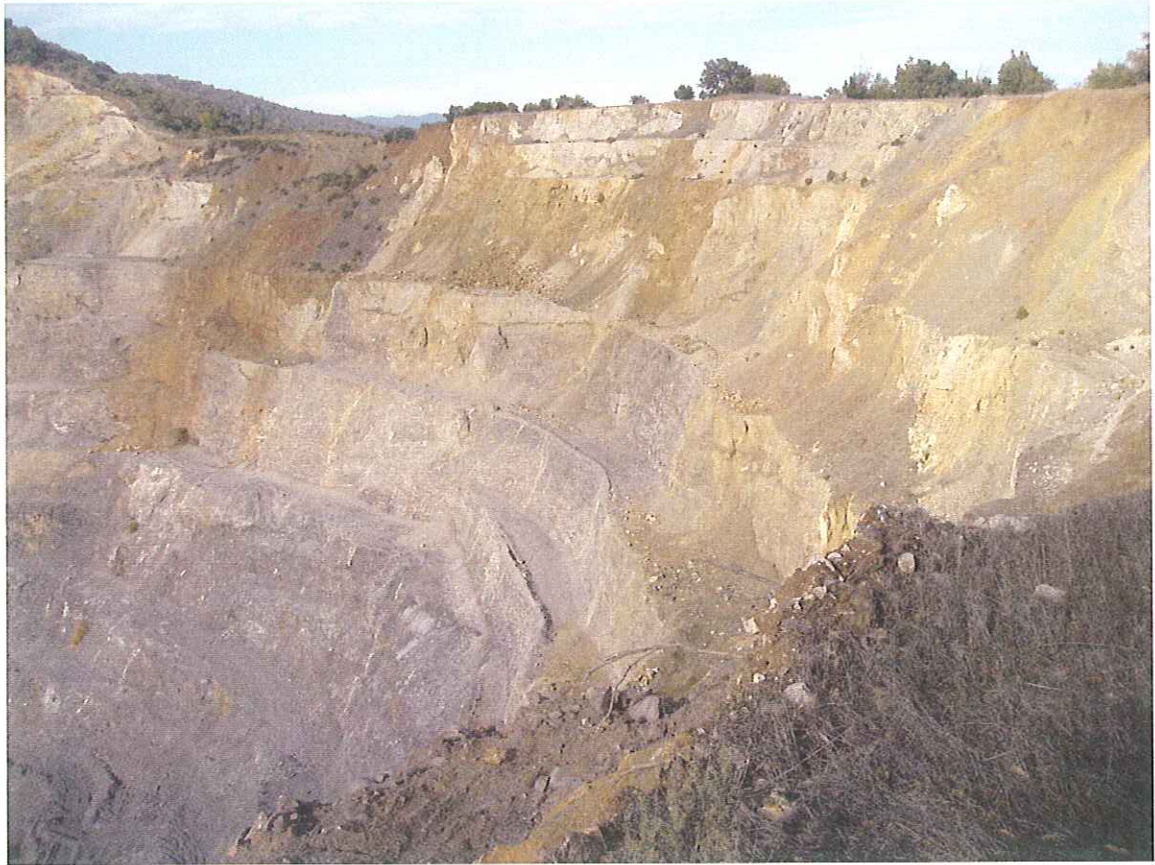
Photo 1. Quarry benches that have not been cleared have accumulated debris from local slope failures.
