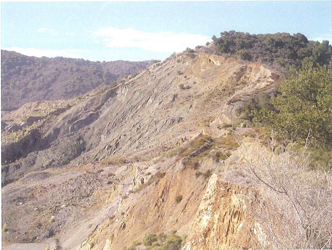
Photo 2. The Main Landslide showing well-defined scarps above the "headscarp" area, indicating ongoing deep-seated failure of the upper portion of the landslide.
