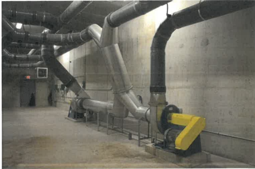
Figure 9: Fan room for SV Composters (ECS, 2015)
