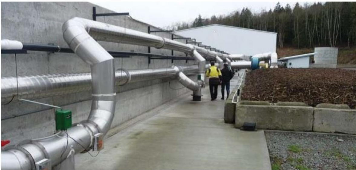
③ CASP Aeration and Biofilter
