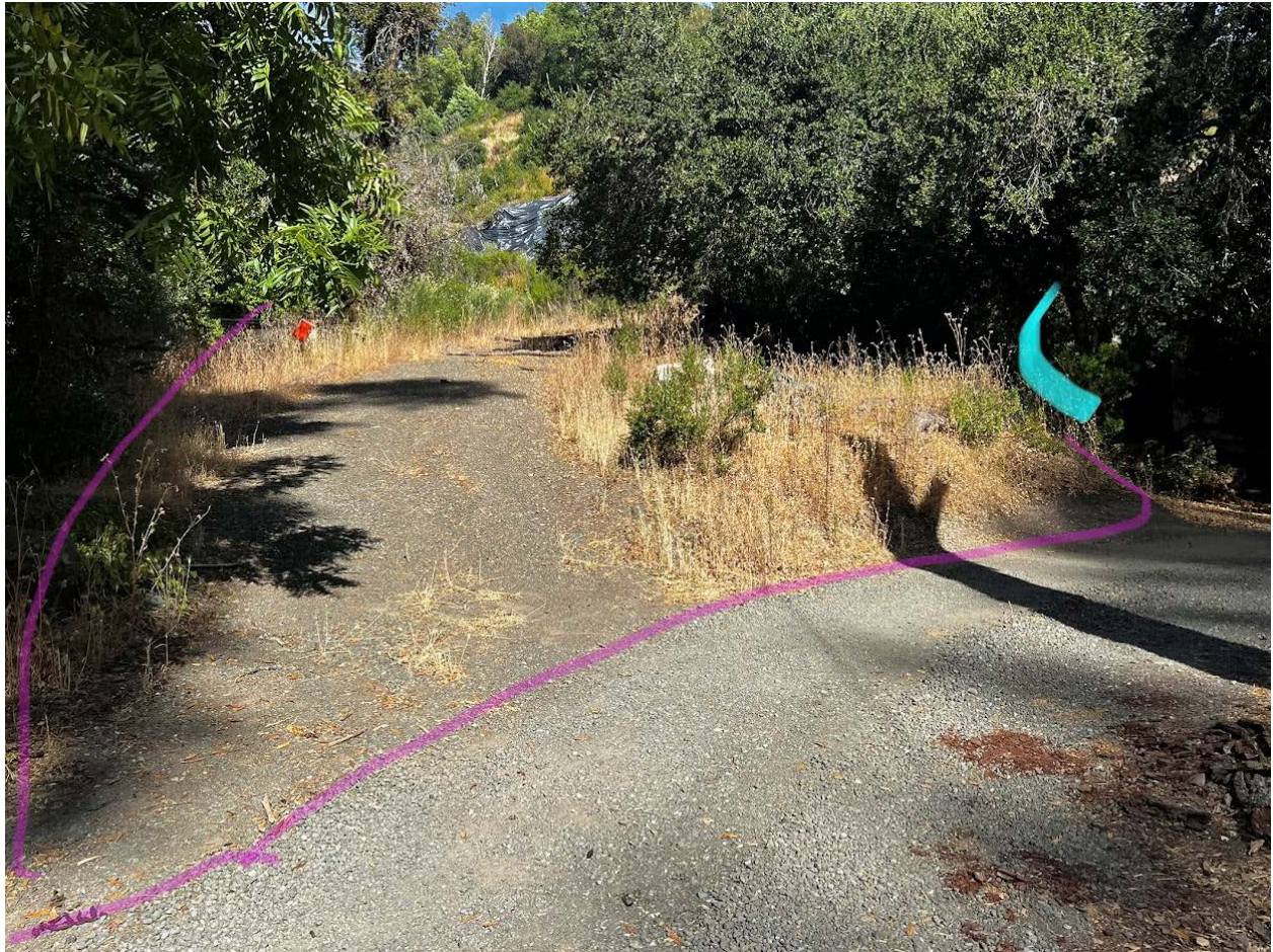
Photo 1. Area bordered in purple has been built up, creating a significant slope. Area in blue is where a retaining wall has been built.
