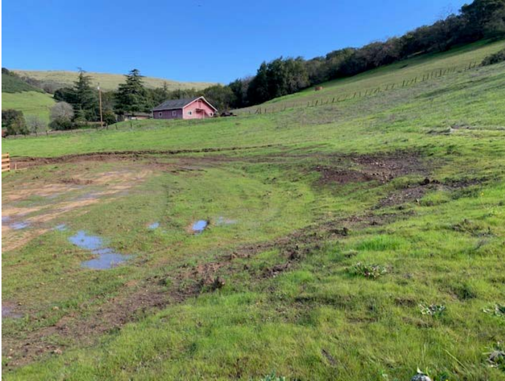
Appendix A-1. Grading Violation-Area 1, February 11, 2019.
