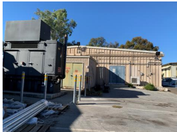
Figure 5: Rear (southeast) façade with flush steel double doors, shed addition and separate electrical equipment structure, looking northwest.
