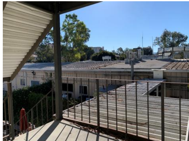
Figure 3: View of covered walkway and rear portion of northeast facade of 333 Bonair Siding Road from landing located at 327 Bonair Siding Road's southwest facade.
