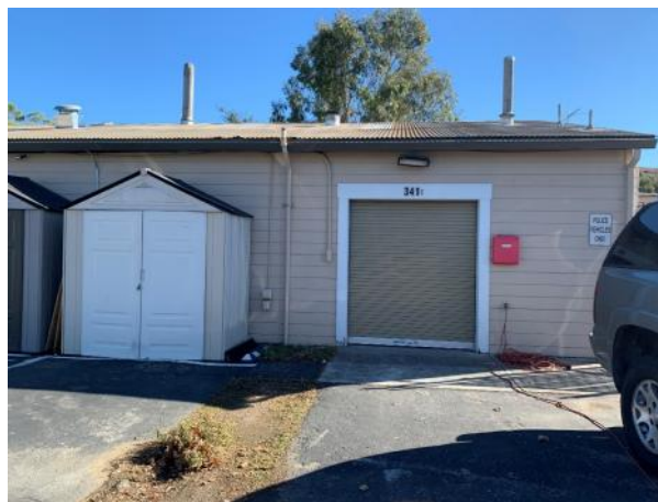
Figure 4: Roll up steel door at garage bay at south end of southwest façade, looking northeast.
