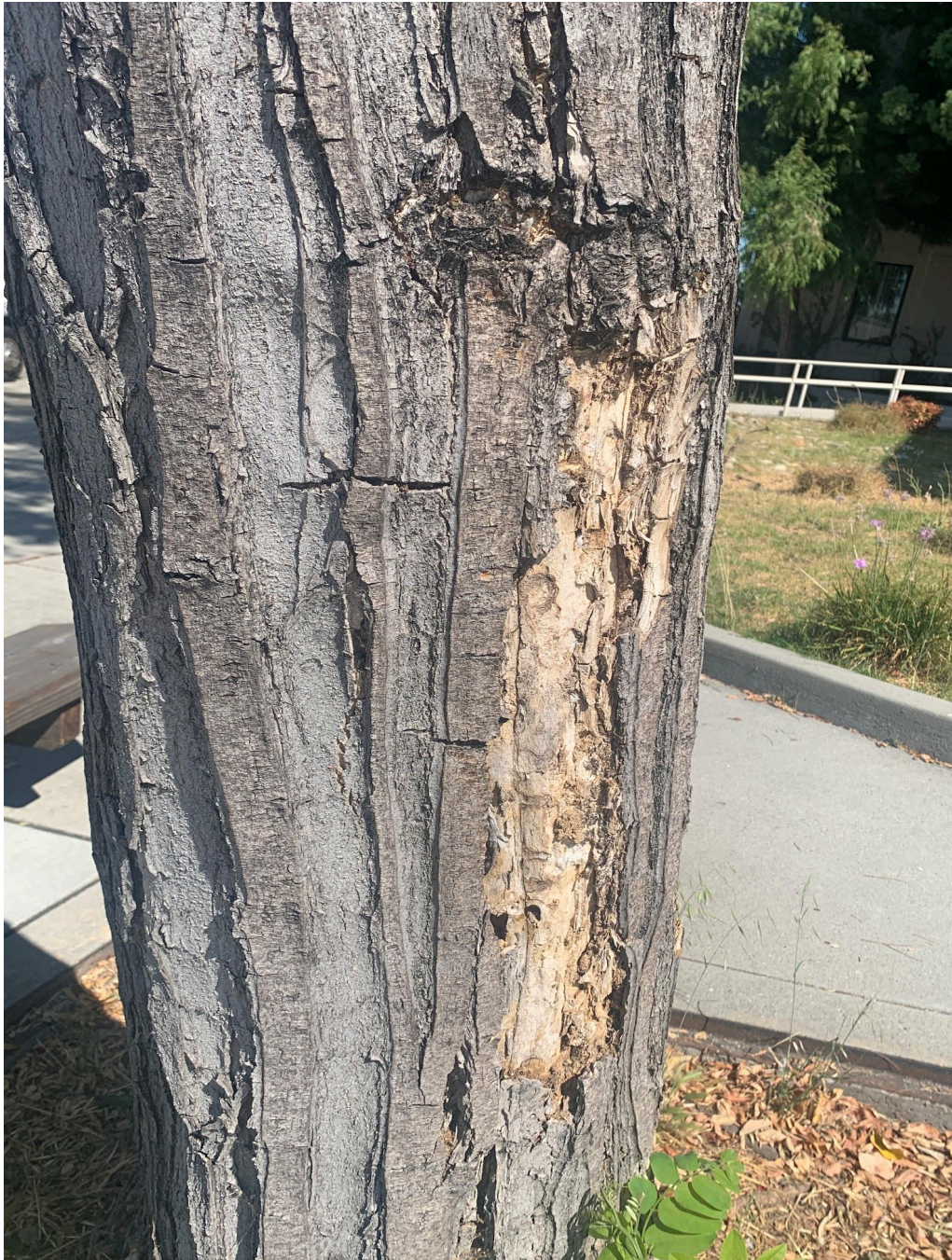
Photo 2. Closer view of the decay in the trunk. There was sounding feedback in the trunk indicating internal decay.
