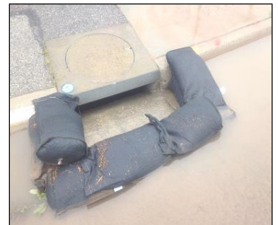
Storm drain inlet protection
