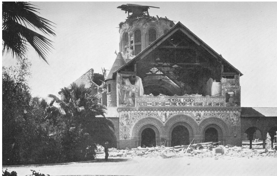
Damage to Memorial Church
