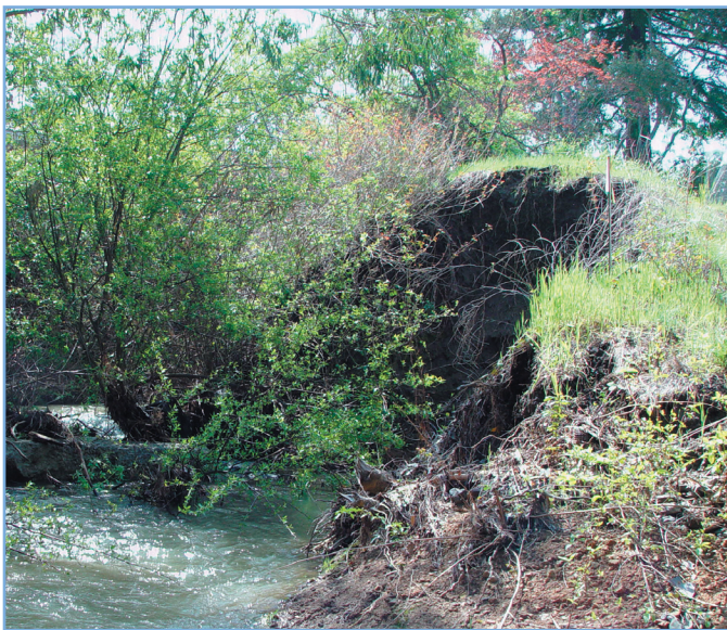
Erosion damage on Adobe Creek.
